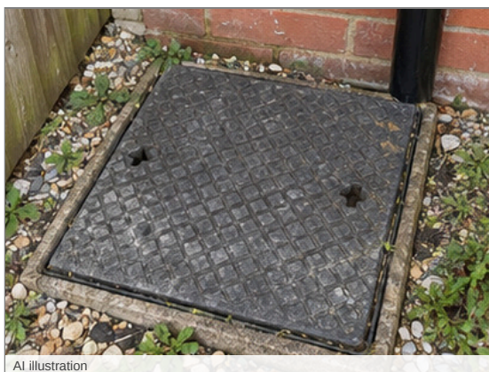
Photo - 87 Rear inspection chamber - no access
