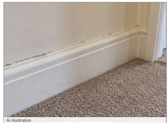
Photo - 52 Skirting board
