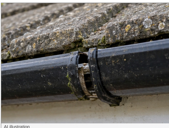
Photo - 16 Open joint
