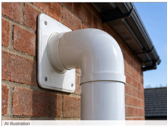
Photo - 77 Boiler flue
