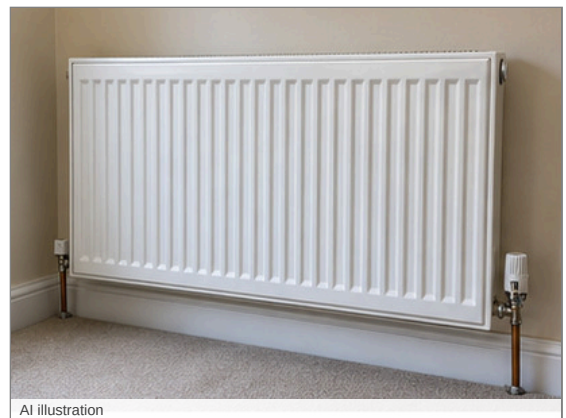
Photo - 78 Typical radiator
