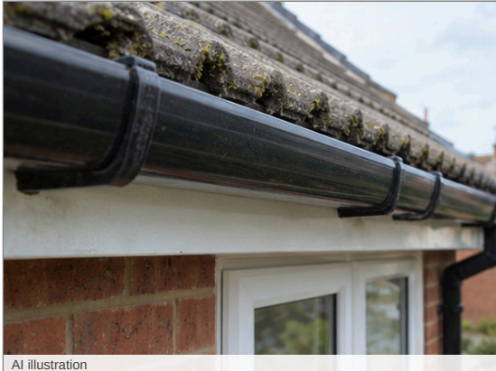
Photo - 12 Front gutter
