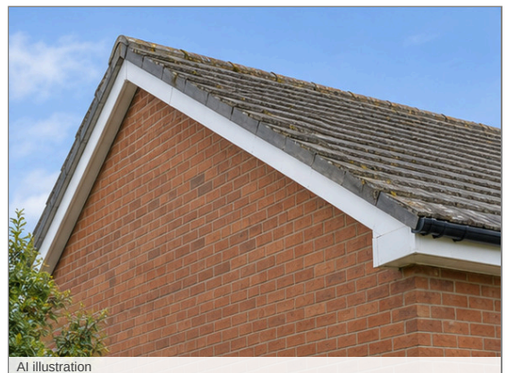
Photo - 10 Undercloak - potential asbestos containing material
