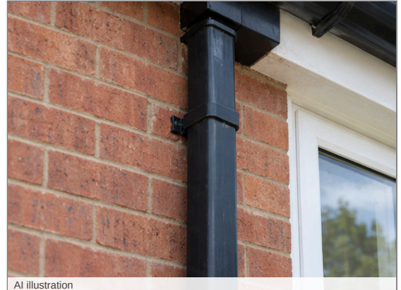
Photo - 13 Front right downpipe - shared
