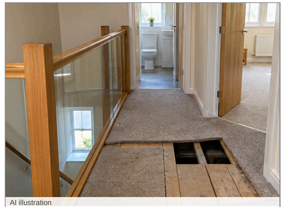
Photo - 45 First floor landing - loose floorboards
