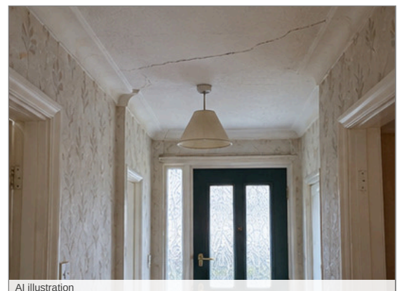
Photo - 68 Entrance hall - minor fracture noted
