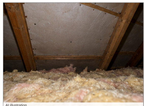
Photo - 70 Plasterboard visible in the loft
