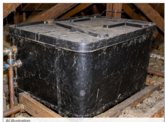
Photo - 111 Primary water tank
