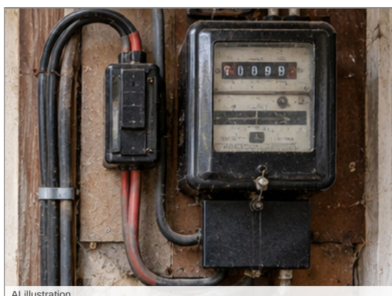
Photo - 101 Incoming main and meter
