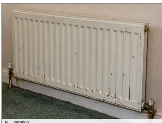
Photo - 115 Typical radiator
