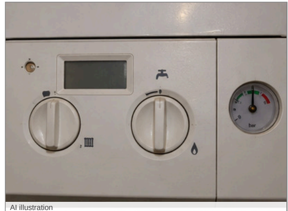
Photo - 118 Boiler controls
