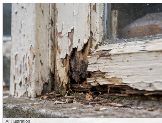
Photo - 52 Rotten frame
