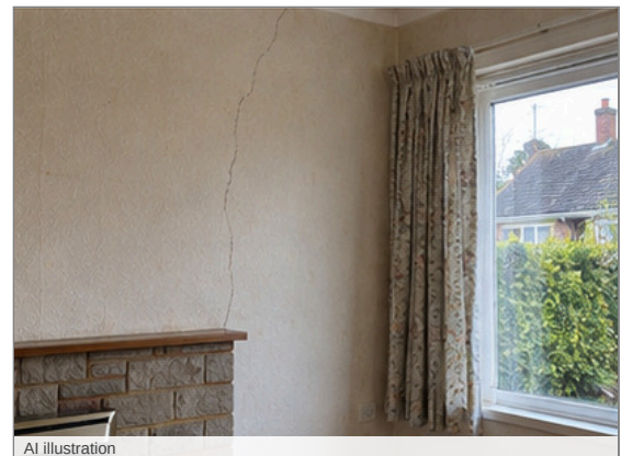
Photo - 74 Living room front elevation - minor fractures noted
