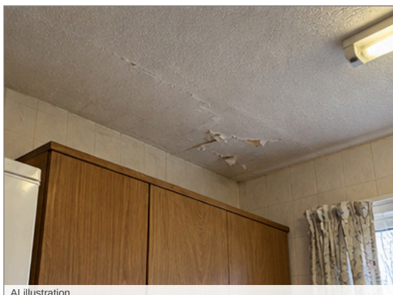
Photo - 71 Kitchen - minor repair required
