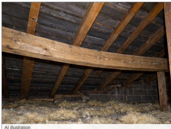
Photo - 64 Rear purlin - moderate deflection
