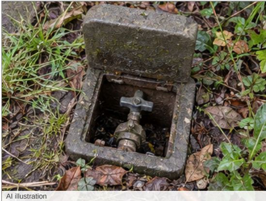
Photo - 106 External stop valve (assumed)
