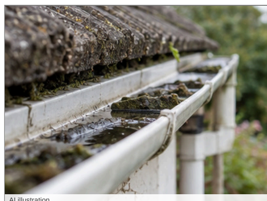
Photo - 22 Incorrect falls
