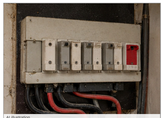
Photo - 102 Distribution board
