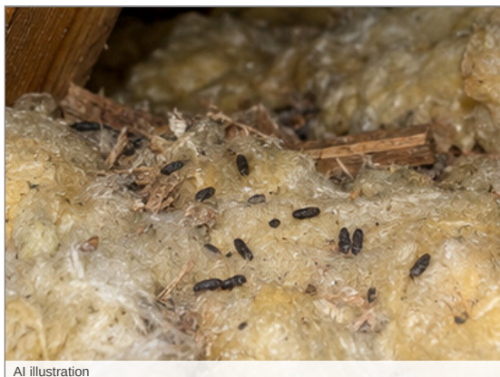
Photo - 66 Evidence of rodent activity
