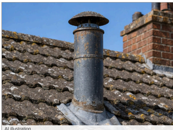
Photo - 113 Boiler flue
