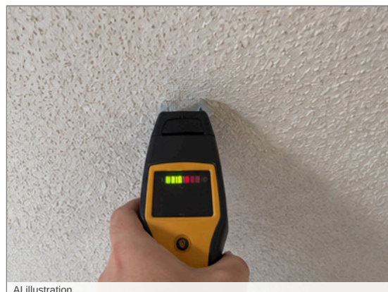
Photo - 72 Low moisture reading
